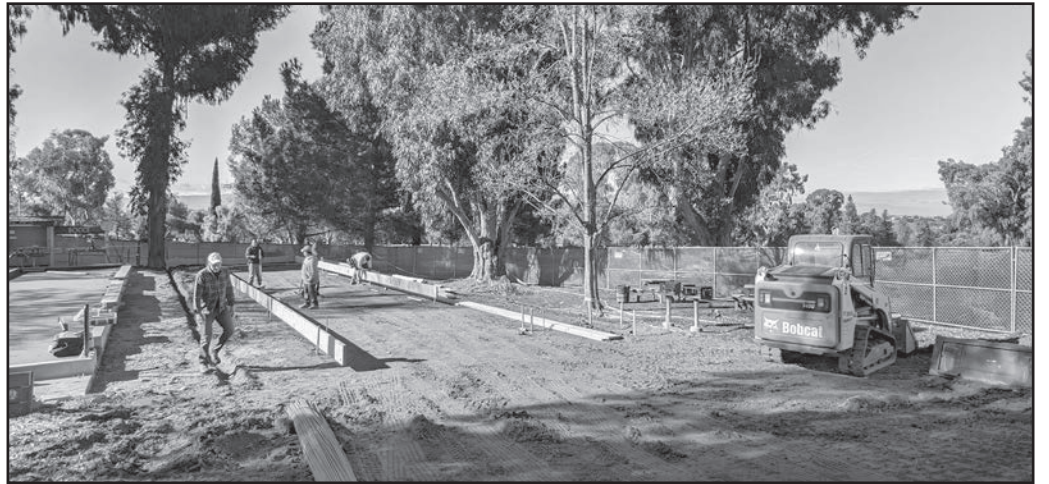
A peek inside the fence: Workers are off to a good start as court #3 takes shape.
