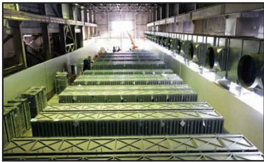
Battery racks sit in former turbine halls at Moss Landing Energy Storage Facility
