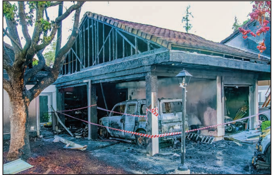
The burned carport on Montgomery Bend. (See page 4 for more fire pictures.) Photo by Frank Langben
