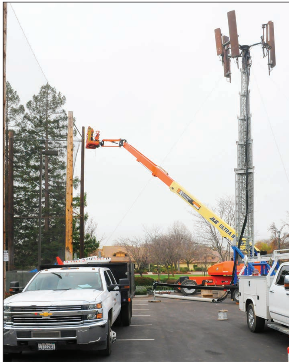
Workers from T-Mobile replace one of the tall driving range poles and prepare to install new equipment. Temporary transceivers are mounted on a truck to maintain T-Mobile cell service while the new transmission equipment is installed on the top of the new pole. The work should continue into February.
