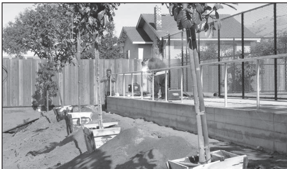
With the major infrastructure in place, Saviano Construction workers install the many various fixtures and landscaping at the Pickleball Courts.
