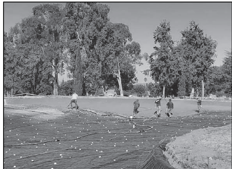
At the golf course lake at Hole #10 California Waterscapes sprays gunnite into the lake basin to prevent the water from leaking into the ground. Soon the lake will be filled, and a new water feature will provide an aesthetic compliment to the lake.
