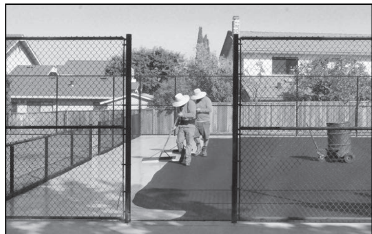
At the Pickleball Courts Construction site, workers from Saviano Construction put a base coat on the courts.
