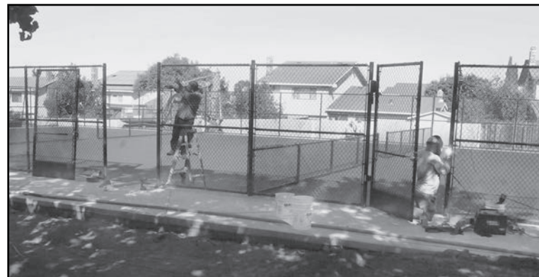
Workers install the gates on the fence surrounding the Pickleball Courts. Construction has been steadily progressing with a late-November completion date as the goal.
