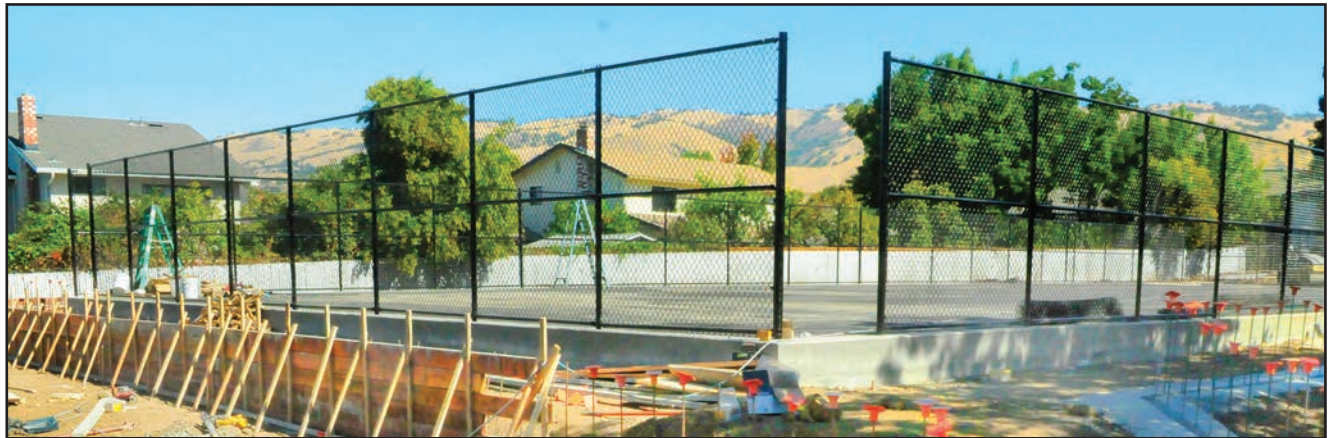
With the playing surface installed, the chain-link mesh was mounted on the fence frames.
