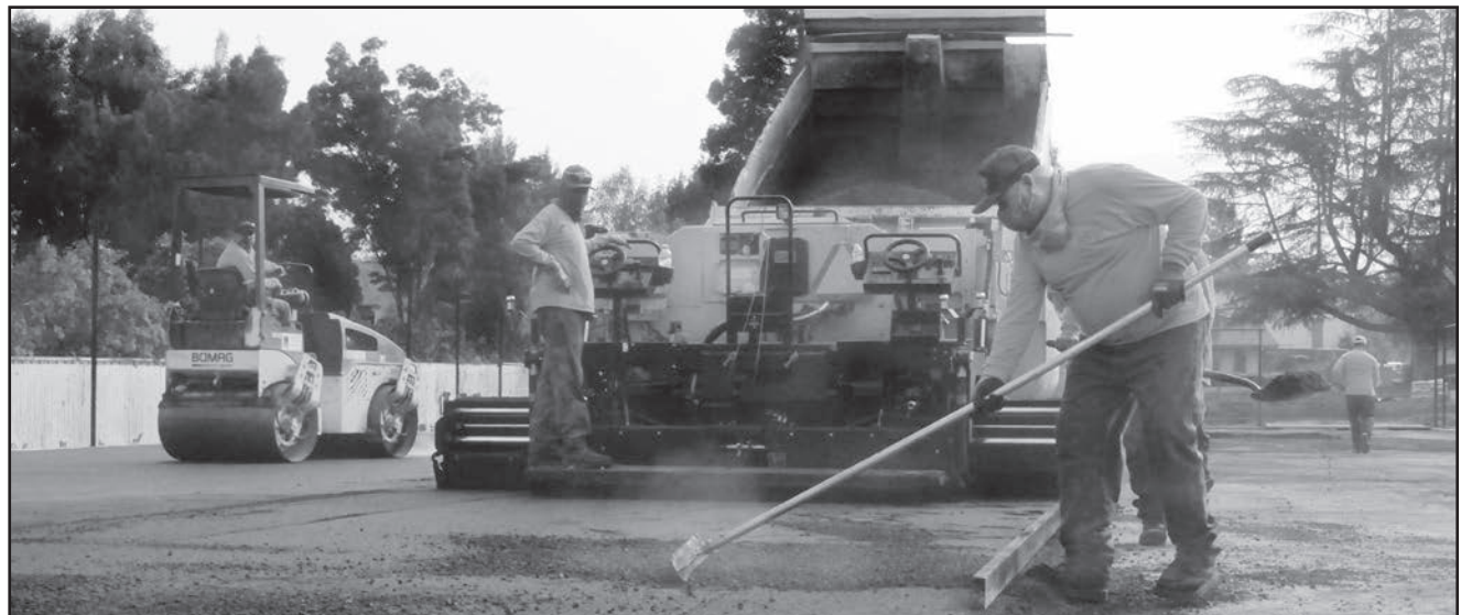
After leveling and packing the underlying soil, the pickleball courts are covered with a layer of asphalt.
